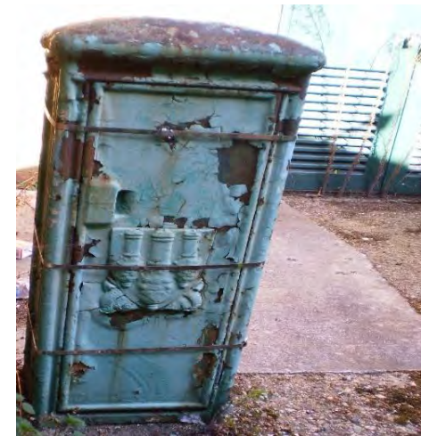
Courtlands Avenue 1960's electricity sub-station with Woolwich's coat of arms
