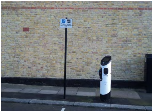
Electric car charging point, Kellerton Road
